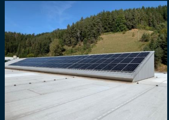
Photovoltaic installation Plant 2 Packaging
